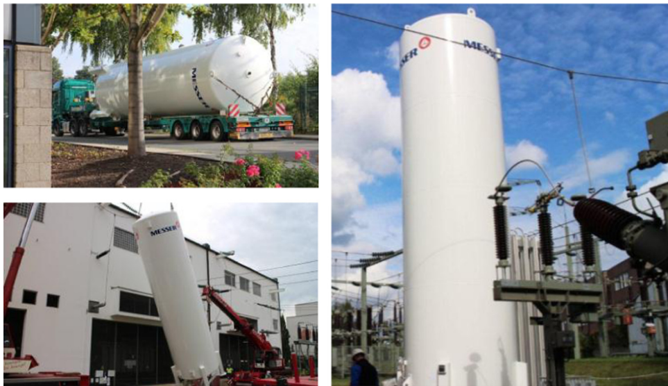
Fig. 5. Cooling RWE substation in Essen, Germany – delivery and installation of the liquid nitrogen vessel.
