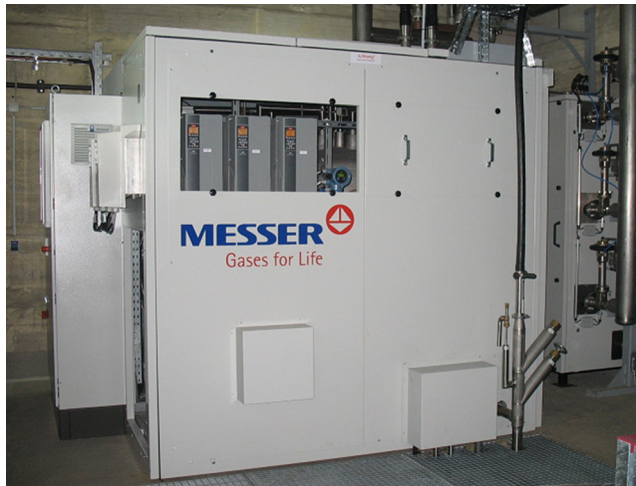
Fig. 6. Cooling unit installed at RWE substation in Essen (Germany), ready for operation.
