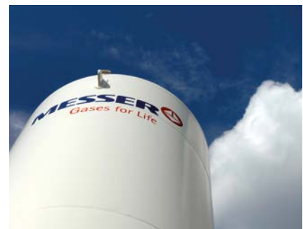
Cold-insulated nitrogen storage tank
